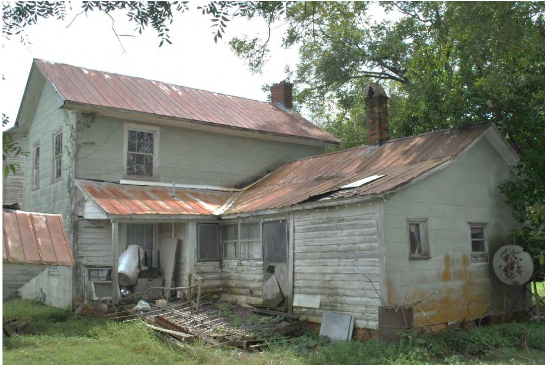
Blackwelder Family House, Original House, Rear (West) Elevation and Rear Ell, Looking Southeast.
