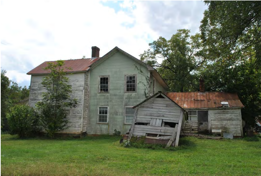
Blackwelder Family House, Side (North) Elevation and Ruinous Well House, Looking South.
